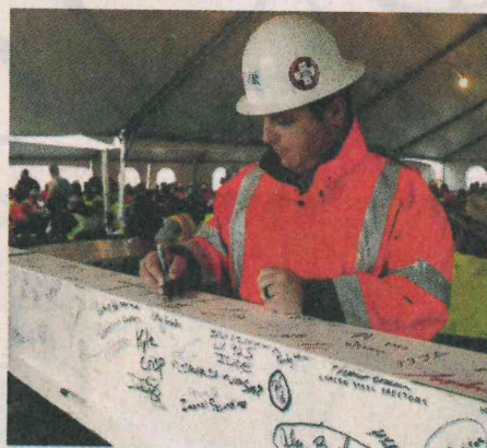
Daniel Vincent, superintendent for DPR Construction, signs his name on the topping-off beam before it is placed in position.
